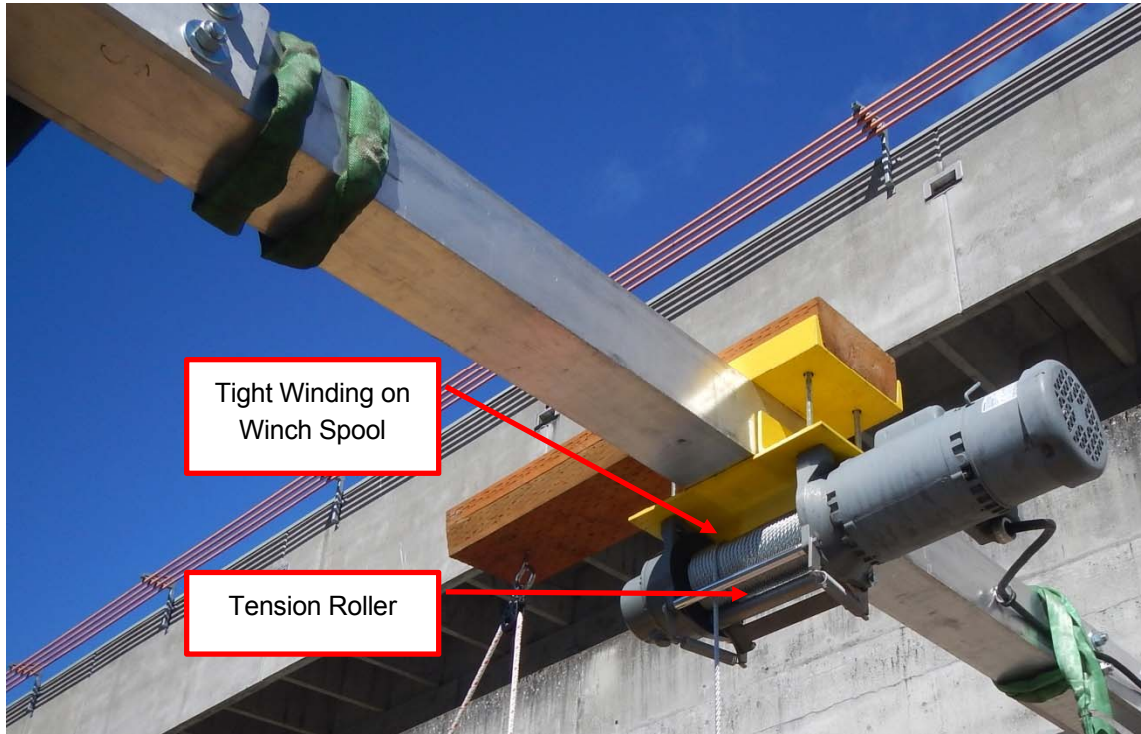
Photo 2-7 Winch Cable Tension Roller
